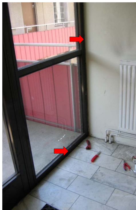
A sealant has been used by the glass section
