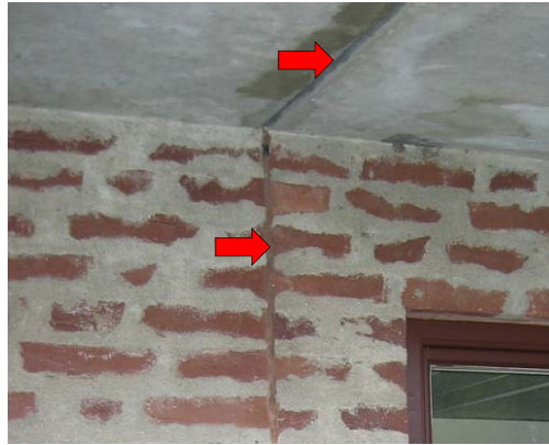
Sealant in an expansion joint in a brick wall and exterior passageway
