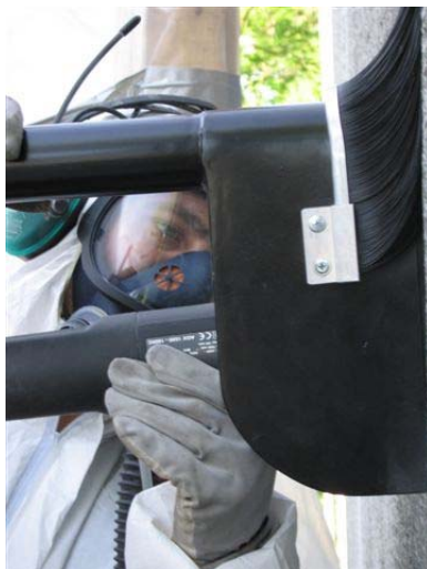
Grinding joint walls with the Milwaukee AGV 16180 QXC grinder, equipped with the SP dust collector.
